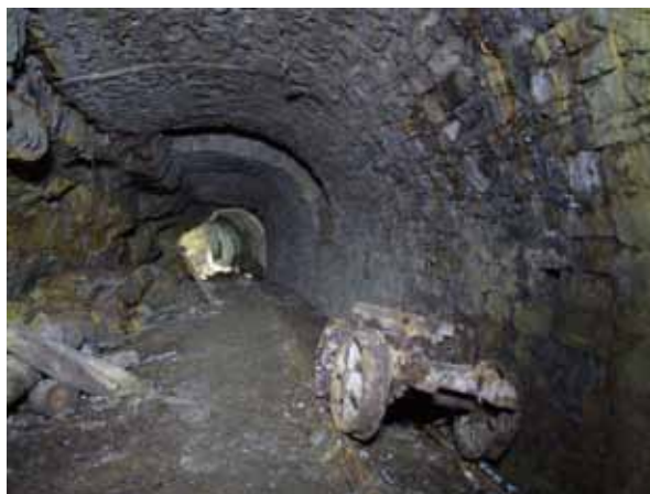
Figure 14.3 Whitewood vein, Rampgill Lead and Zinc mine, Nenthead, Cumbria. Horse level roofed with sandstone dry arching. Floor heave caused by later undermining. Abandoned mine wagon end tipping chassis. Last worked 1922. © James Heaton
