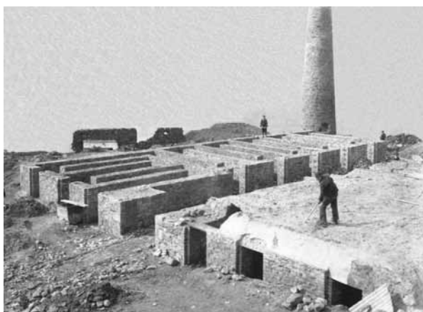
Figure 12.4 Arsenic flues attached to the calciner at Botalack, St Just, under construction in 1907. © Pete Joseph
