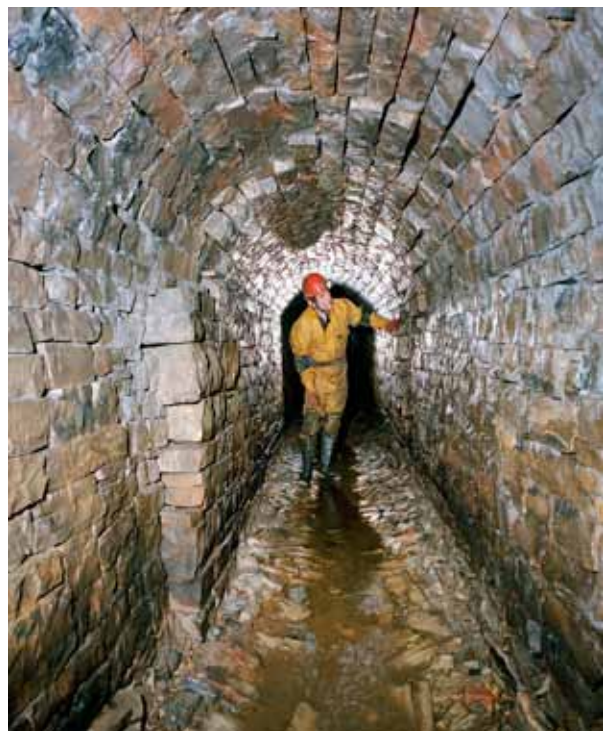
Figure 14.1 Drystone arching of 1861-62 in the Main Level at East Ecton Mine, Staffordshire. © Paul Deakin
