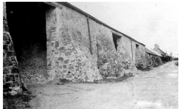
Figure 6.8 The buttressed wall of a ball clay cellar at Teignbridge in Devon. © BCHS
