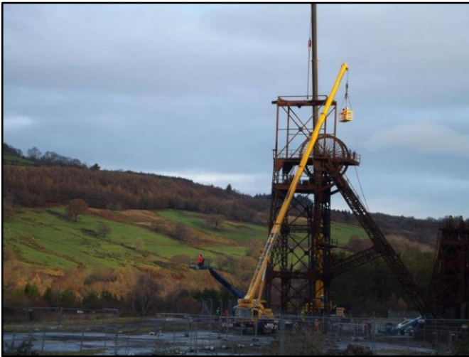
Work underway on Cefn Ceod Colliery headframes. Photograph courtesy of Keith Davies, Museum Manager
